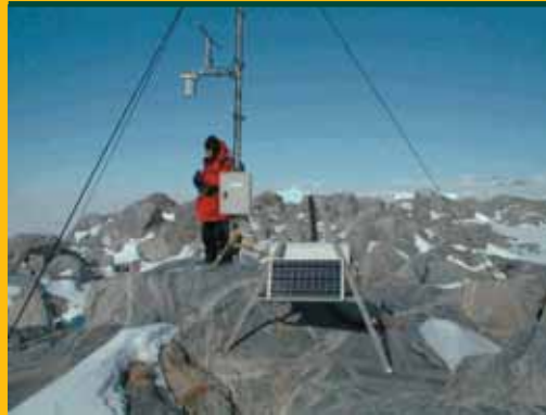
This clear day at Cape Roberts belies the extreme weather that often pounds the tide gauge's batteries, sensors and other hardware.
