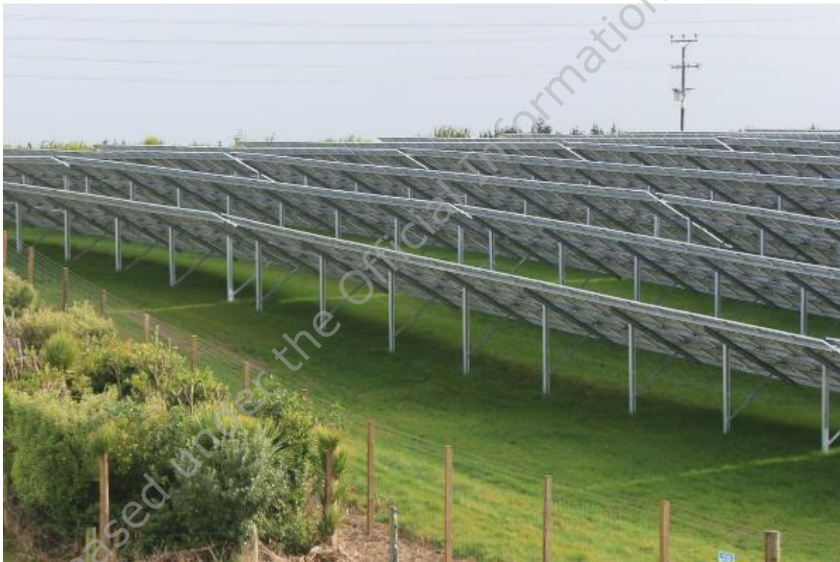
Figure 2: Kapuni Solar farm, Taranaki showing solar panels erected on mounting structures with grass growth underneath and around the solar panels.
