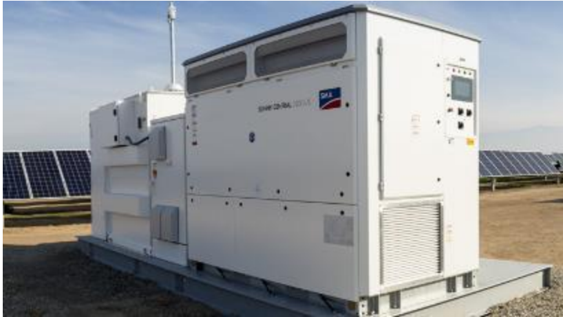
Figure 3: Example of a skid mounted inverter station
