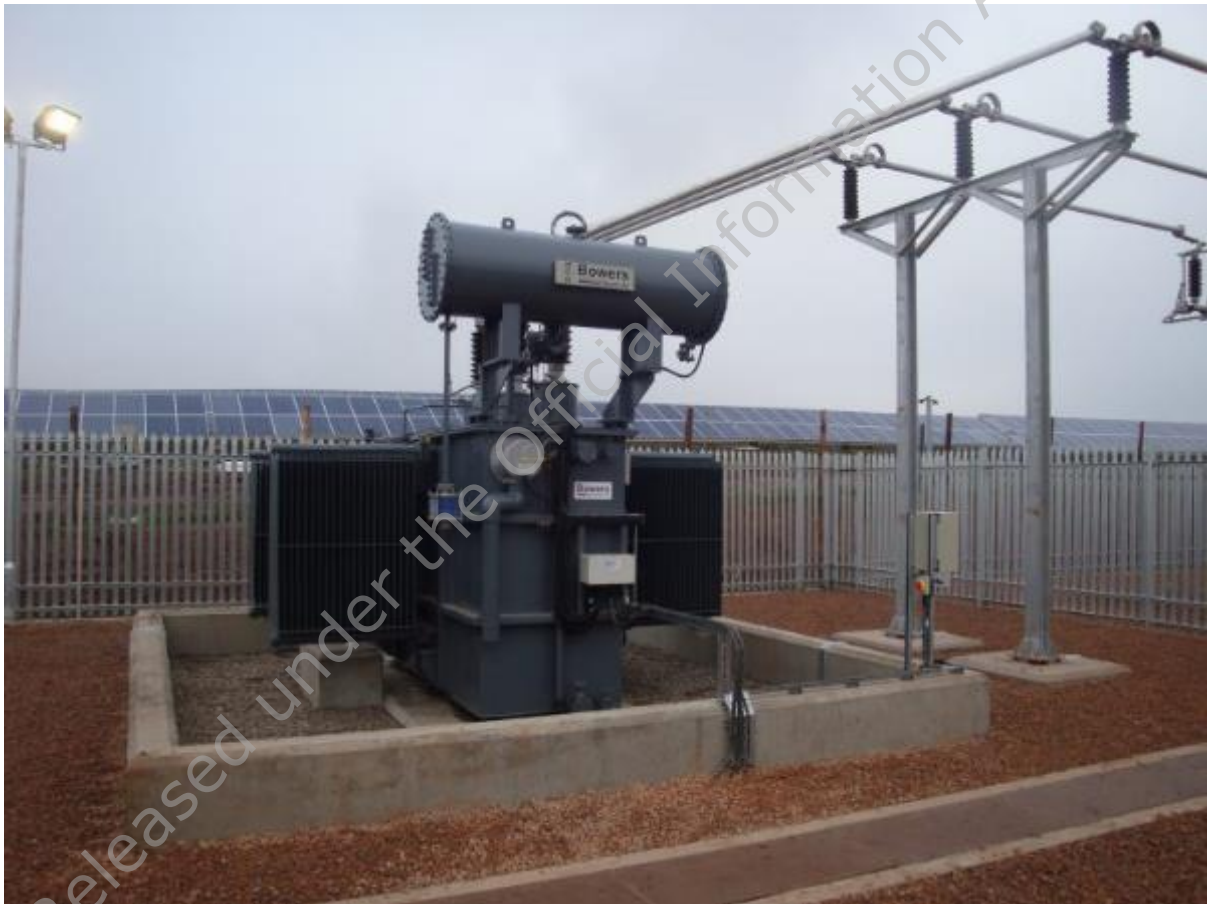
Figure 4: Example of switch yard / room
