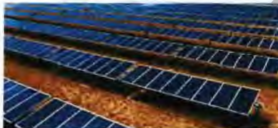
Figure 4 - Solar arrays in a Solar Farm
