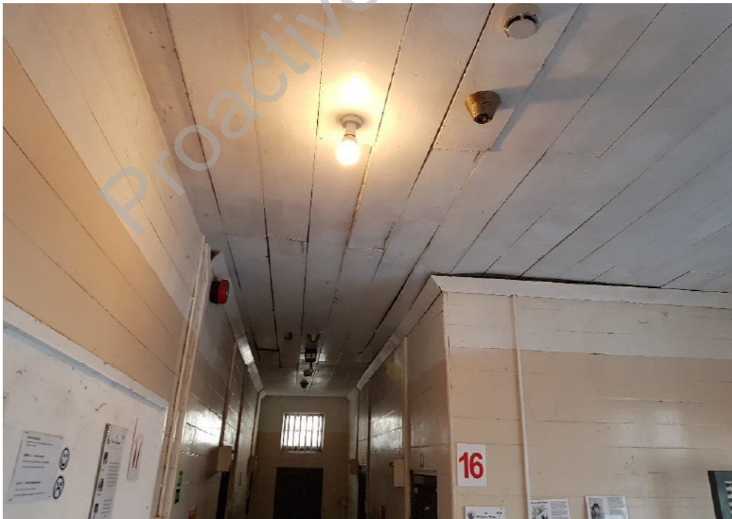
Figure 11: Timber staking boards for the internal wall and ceiling lining of the main prison block (Building 4).
