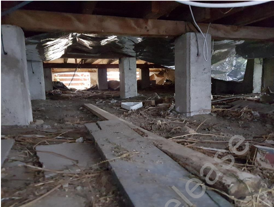
Figure 2: Underneath the timber framed buildings that consist of suspended timber floors on concrete piles.
