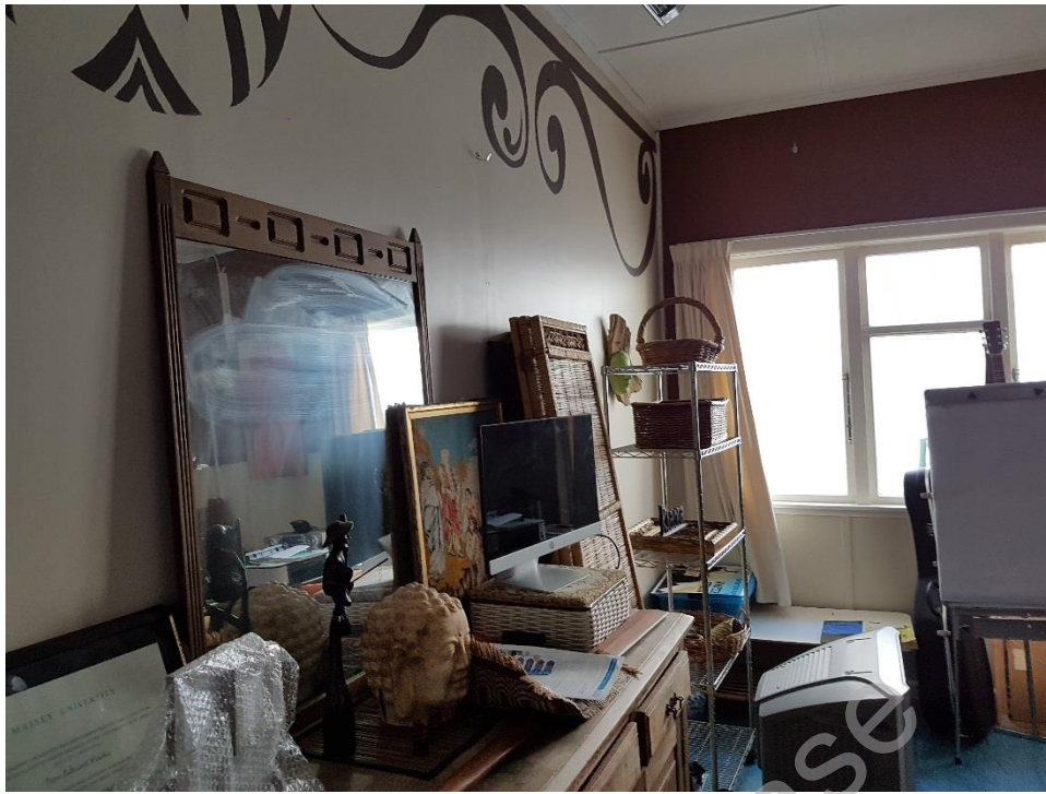
Figure 6: Internal partition wall (timber framed) up to ceiling joists installed in 2003. The wall is lined with Gib Board.
