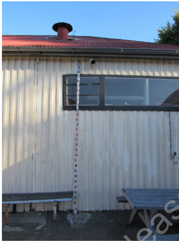
Figure 12: Timber board cladding for the external wall lining at the main prison block.
