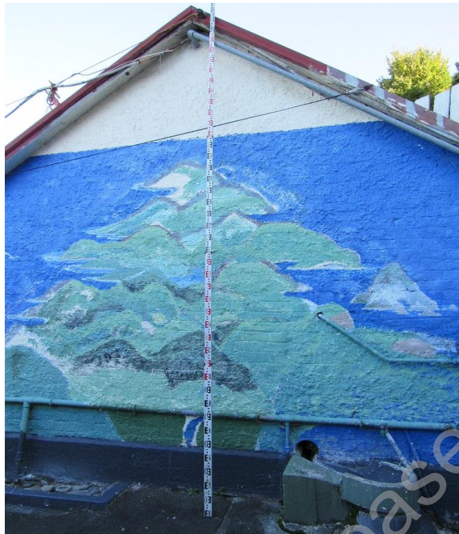
Figure 4: Concrete block wall at the base of the building - around the perimeter.
