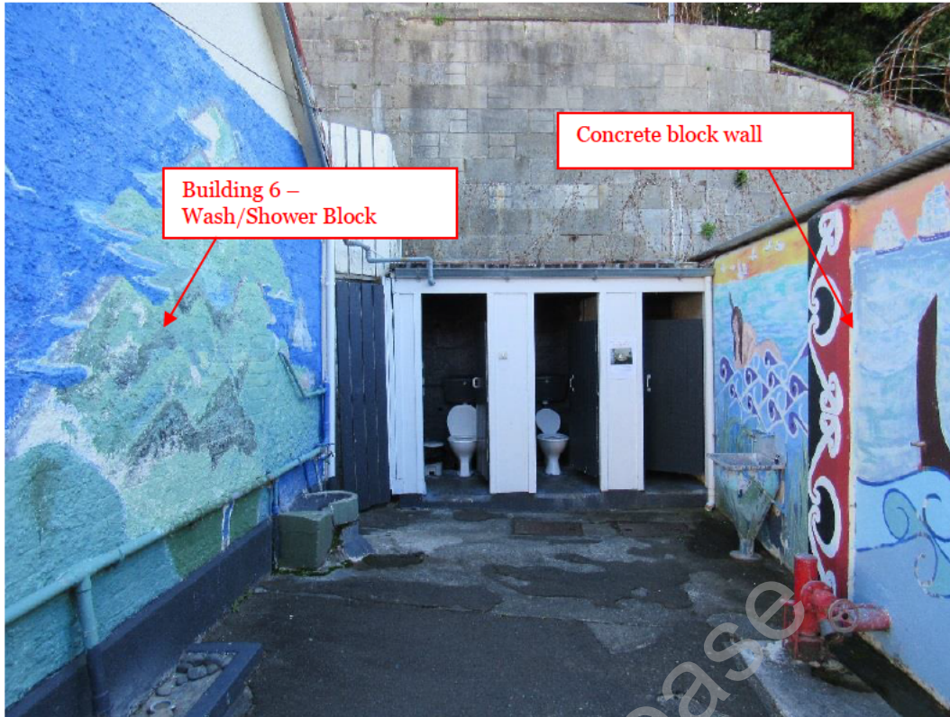
Figure 10: External view of the concrete block wall adjacent to the main office block and opposite to Building 6.
