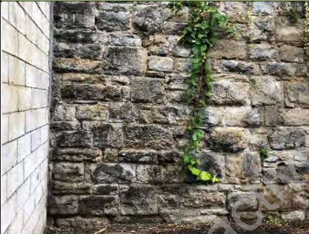
Photo 3) Cracking observed in wall face.
