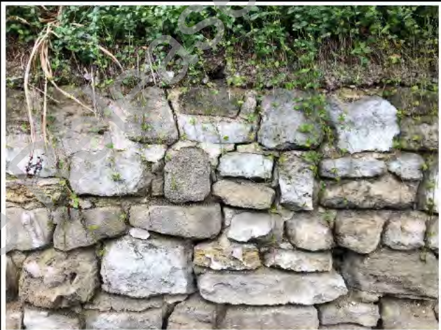
Photo 4) Cracking observed between stone blocks.
