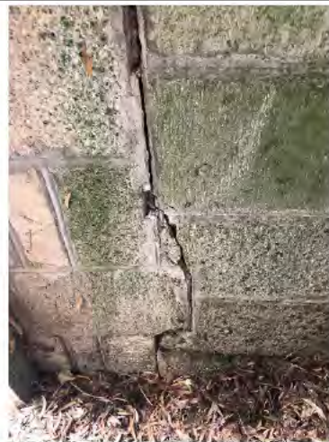
Photo 6) Cracking observed at base of wall.
