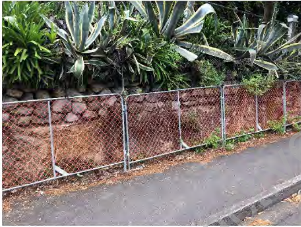
Photo 3) Loose blocks and partial collapse of wall.
