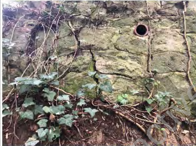
Photo 3) Cracking observed in wall face.
