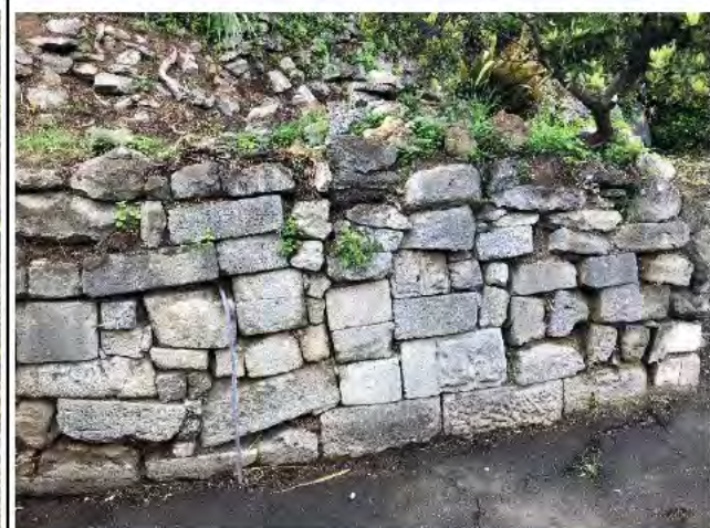
Photo 6) Loosely stacked rocks of wall face.
