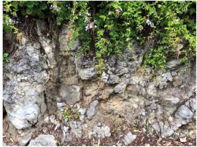
Photo 2) Exposed soil face showing evidence of erosion.
