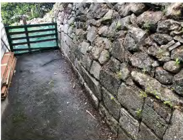
Photo 5) Bulging of wall observed.
