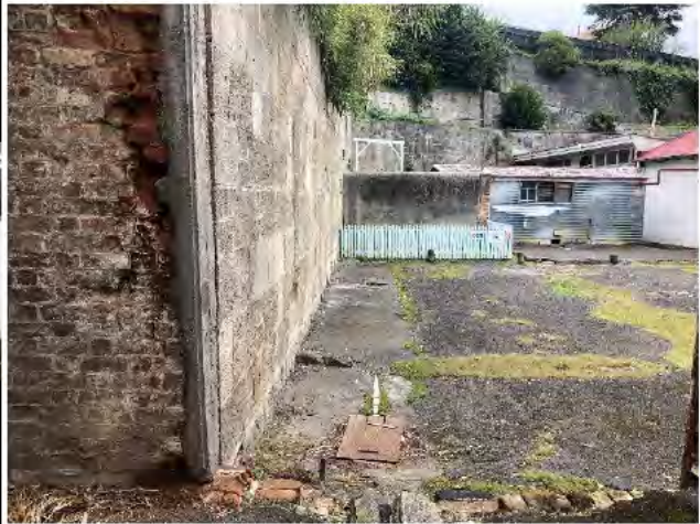
Photo 2) Brick masonry at cracking observed at end of wall.
