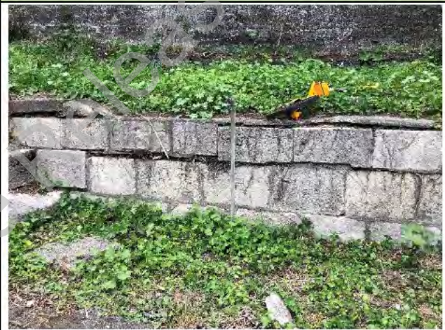
Photo 4) Loose/dislodged blocks observed.
