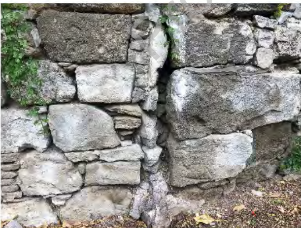
Photo 5) Large displacement/gaps observed in wall. Note old tree root at toe of wall.
