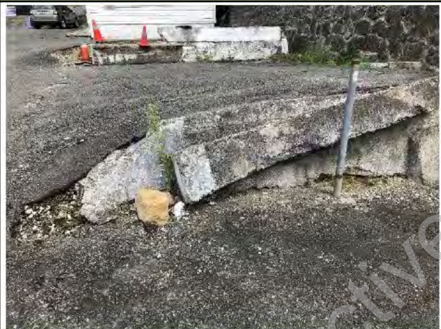
Photo 3) Cracking and top barrier broken off top of wall.
