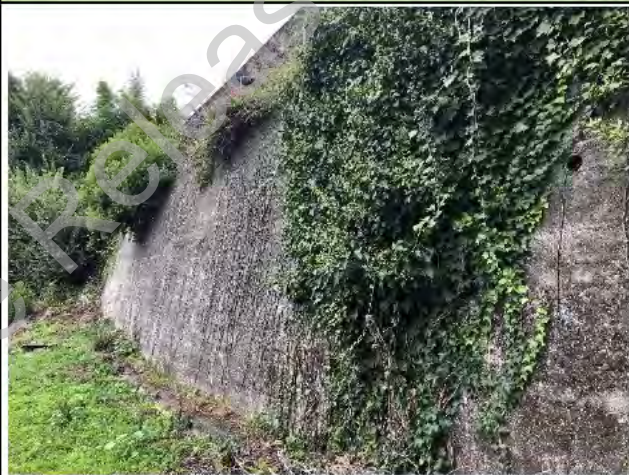
Photo 4) Vegetation growth over face.
