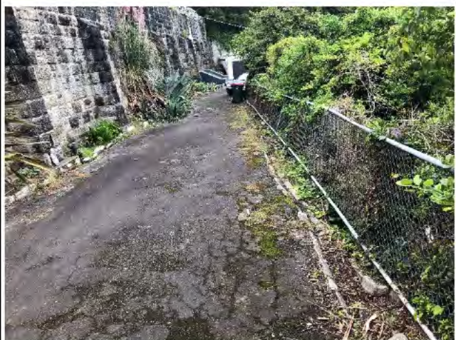
Photo 6) Cracking of access way and rotation of fence at top of wall.
