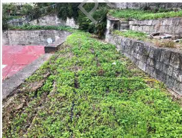
Photo 5) ~300mm wide ground cracks observed at the top of the wall.
