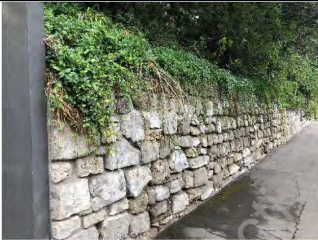
Photo 3) Loose blocks/mortar eroded between blocks.
