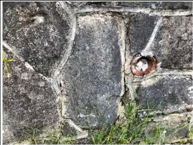
Photo 3) Cracking observed around blocks.
