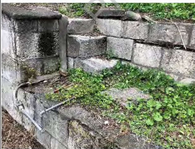
Photo 5) Loose/dislodged blocks observed. Possible wall settlement resulting in "gap".
