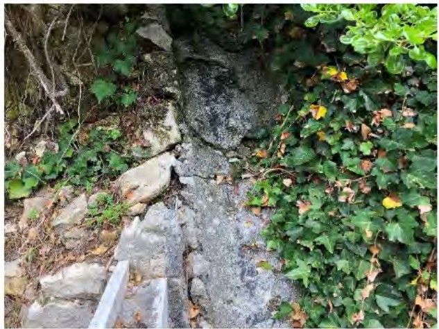
Photo 6) Significant cracking and degradation of upslope concrete channel.
