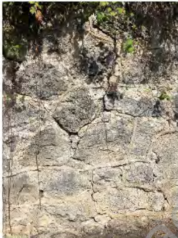
Photo 3) Cracking observed in wall face.
