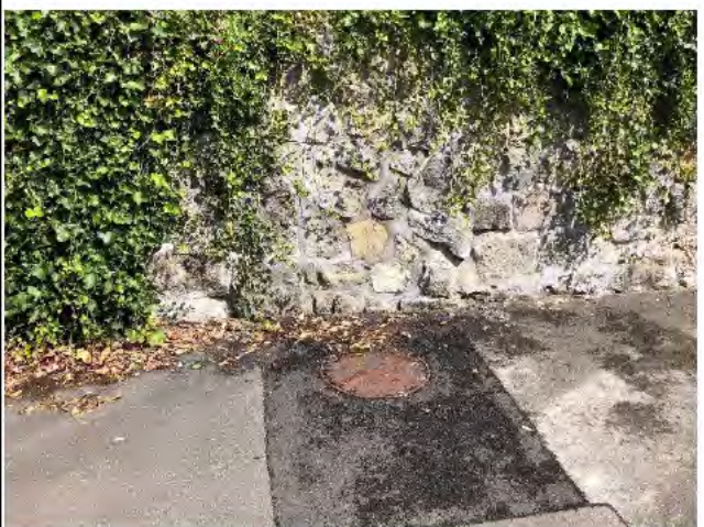
Photo 6) Section of wall appears to have been re-grouted recently.
