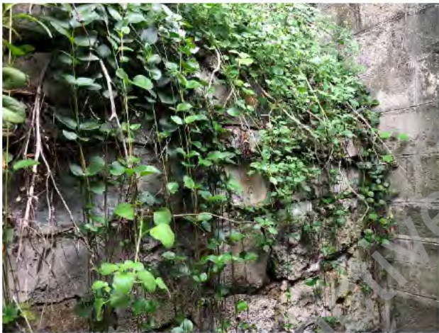
Photo 3) Vegetation observed at top of wall. Cracking and erosion of mortar and blocks.
