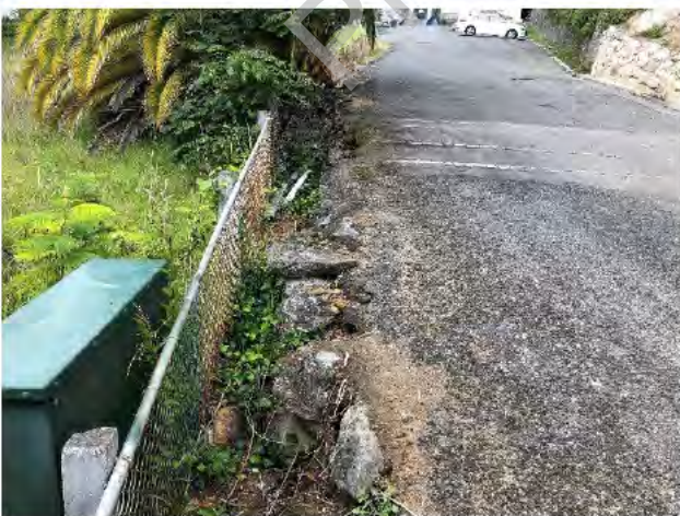
Photo 5) Power box observed in front of wall.
