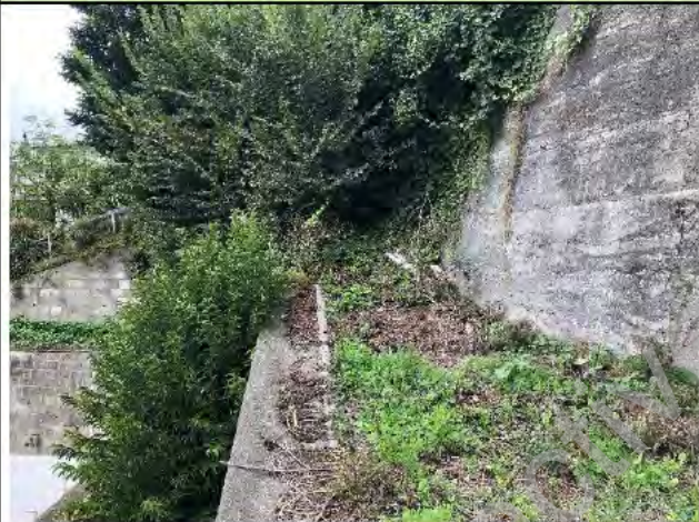
Photo 3) Heavy vegetation above top of wall.
