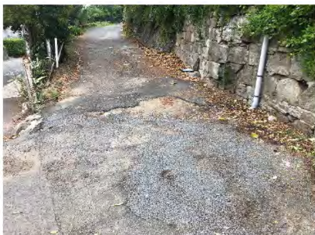
Photo 6) Site driveway/entrance showing PVC pipe outlet and erosion of soil/asphalt.
