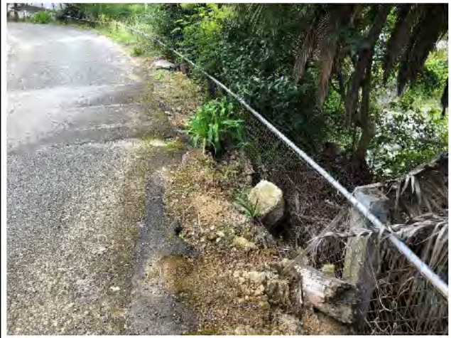
Photo 2) Partial collapse of wall with soil and rock pushing against fence.
