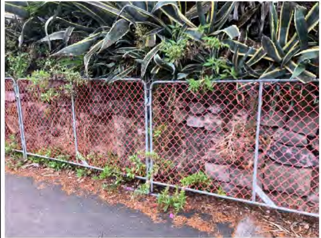
Photo 2) Loose, dislodged blocks and partial collapse.
