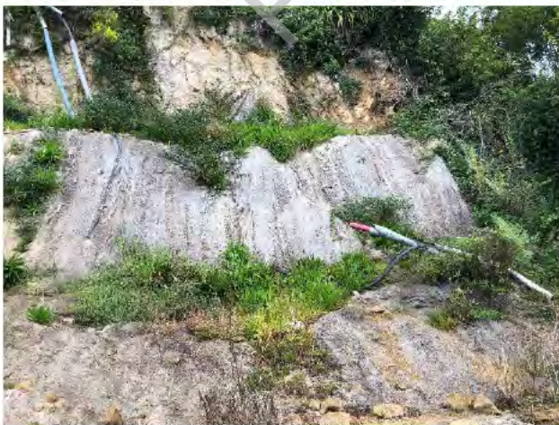
Photo 5) Coconut matting placed over slope following slip. Note protruding, broken services.
