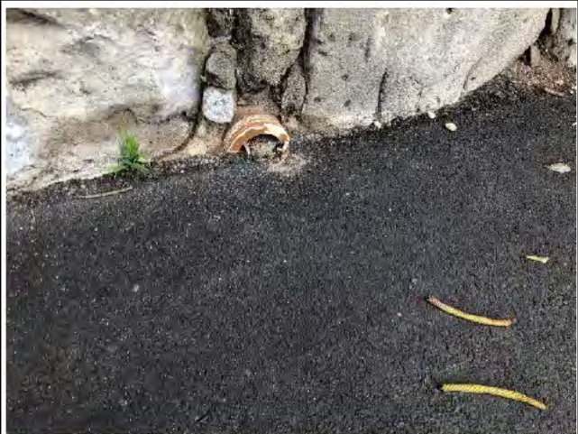
Photo 6) Old drainage pipes appear to have been recently asphalted over in places.
