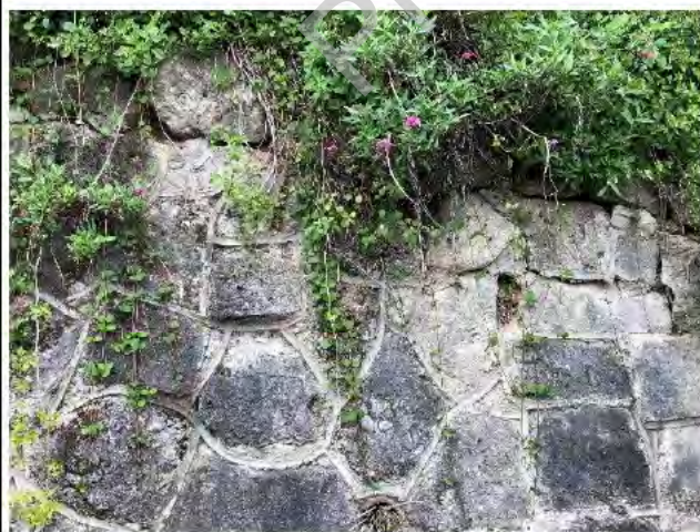
Photo 5) Cracking at top of wall where heavy vegetation present. Root growth through drains.
