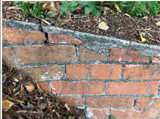
Photo 4) Cracking observed in brick masonry.
