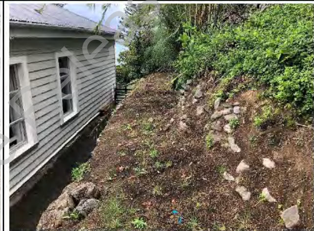
Photo 4) Top tier of wall almost completely collapsed.
