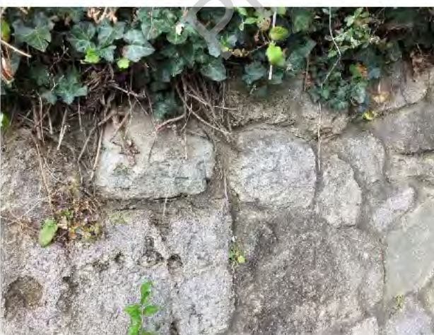
Photo 5) Cracking observed in mortar between blocks.
