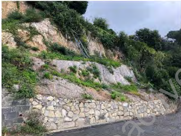
Photo 3) Benched slope covered with coconut matting following slip.
