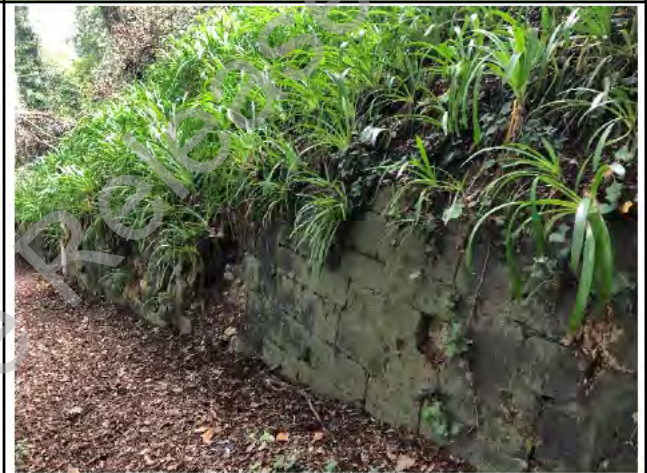
Photo 4) Cracking and partial collapse of wall observed.
