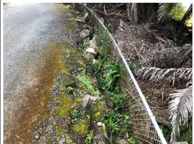
Photo 6) Vegetation and partial collapse of wall.
