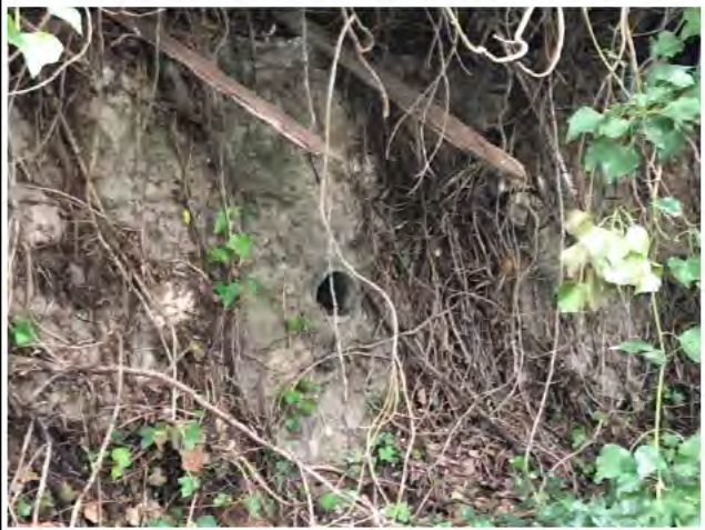
Photo 2) Drainage pipe observed.
