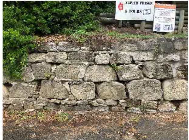
Photo 2) Loose, dislodged blocks.
