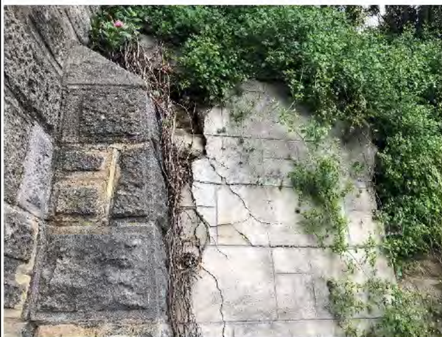
Photo 6) Cracked and partially collapsed façade. Note prison wall on left.
