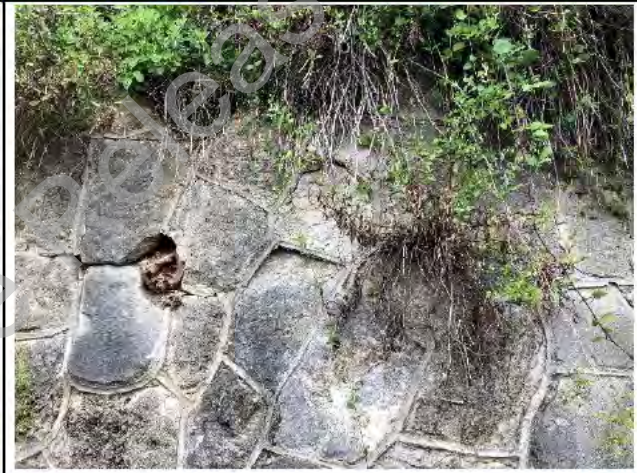
Photo 4) Cracking and broken drainage pipes observed.
