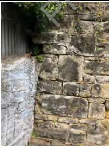
Photo 5) Erosion of stone blocks and mortar observed.
