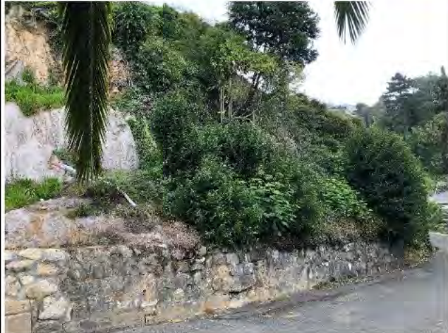
Photo 2) NAP-PRIS-05 view. Note heavy vegetation above wall.
