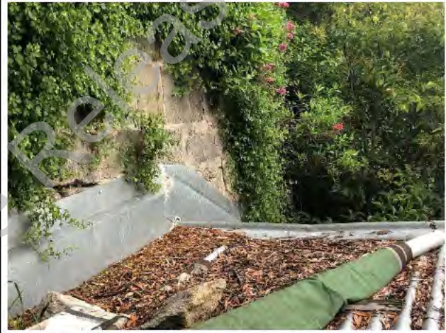
Photo 4) Cracking and observed in wall face.
