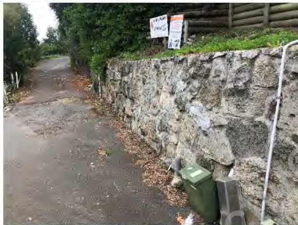
Photo 3) Power box and services in front of wall.
