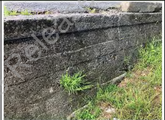
Photo 4) Cracking observed in wall face.
