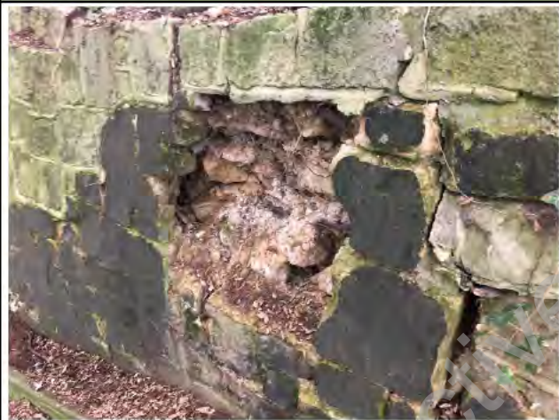
Photo 3) Cracking and partial collapse of wall observed.
