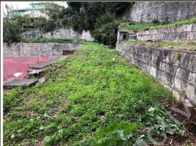
Photo 3) Ground cracking observed in front of wall (behind NAP-PRIS-RW10)
