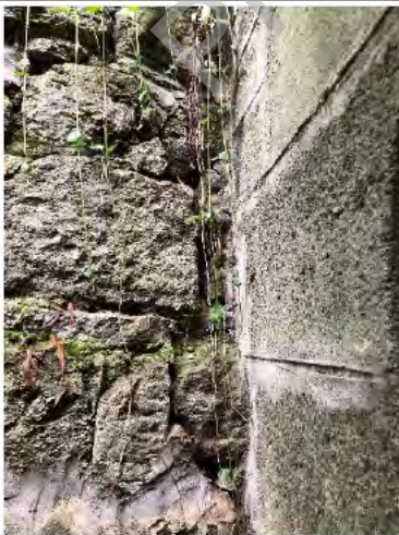
Photo 5) Cracking observed at end of wall.
