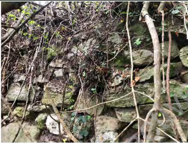
Photo 3) Loose blocks and partial wall collapse.
