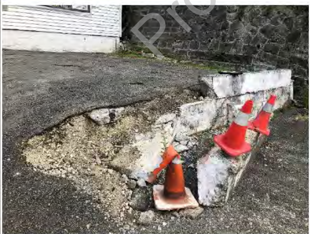
Photo 5) Erosion, wall collapse and broken top barrier.
