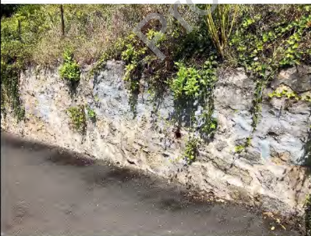
Photo 5) Section appears to have been re-mortared recently.
