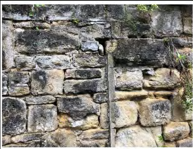
Photo 6) Erosion of stone blocks and mortar observed.
