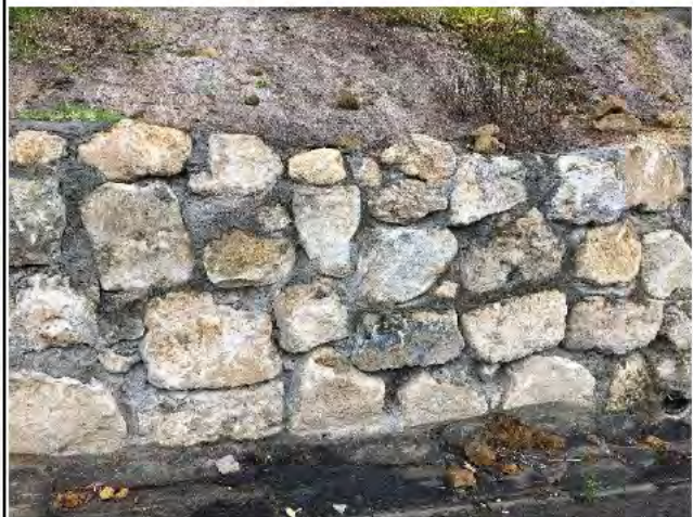
Photo 2) Cracked and missing mortar between blocks.
