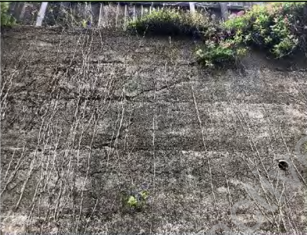
Photo 3) Some cracking observed in wall face.
