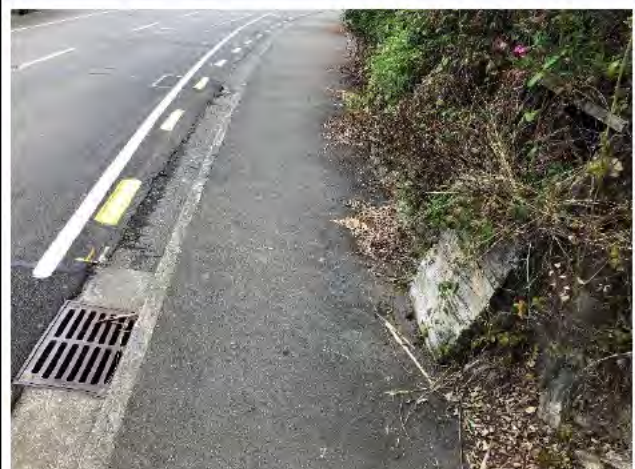
Photo 6) Inferred old stormwater channel observed in wall face.
