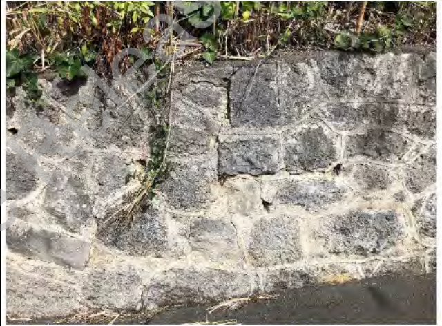
Photo 4) Cracking observed in wall face.
