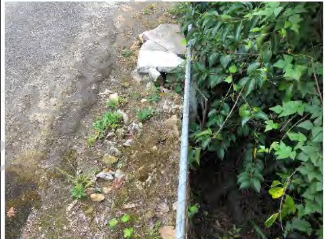
Photo 4) Soil in "channel" pushing against steel mesh fence.
