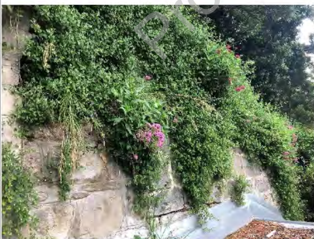
Photo 5) Cracking and vegetation growth through wall face.
