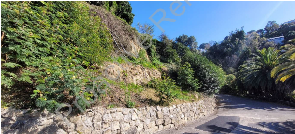
Photo 6 – Existing slip above the driveway.
