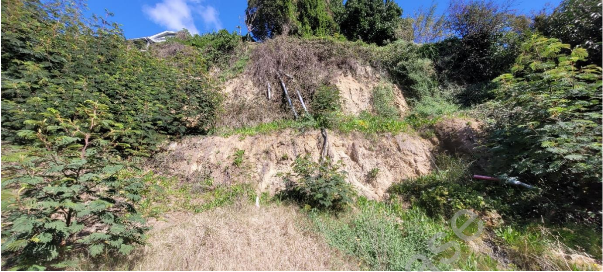
Photo 7 – Existing slip above the driveway.
