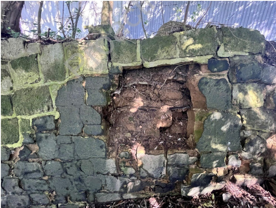
Photo 4 – Section of damage at RW19. Photo taken 03.03.2023, looking west.
