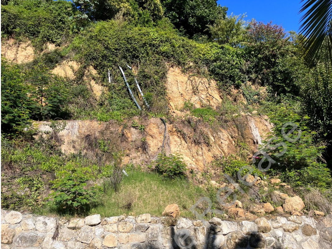
Photo 1 – Rockfall debris above RW6. Photo taken 03.03.23, looking west.
