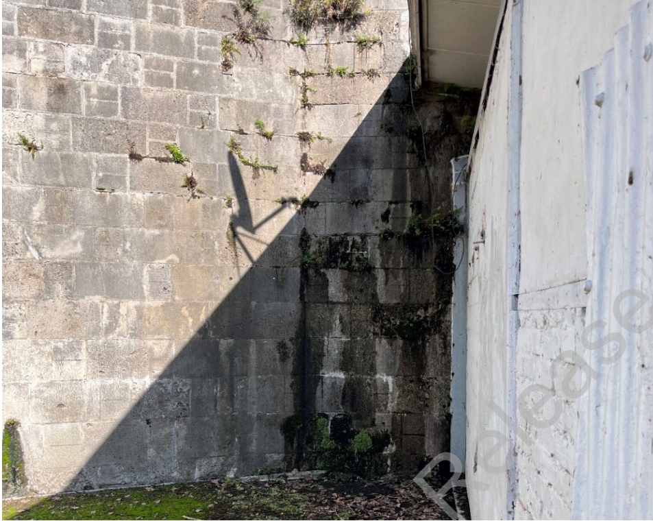
Photo 3 – Seepage from RW10. Photo taken 03.03.23, looking west.
