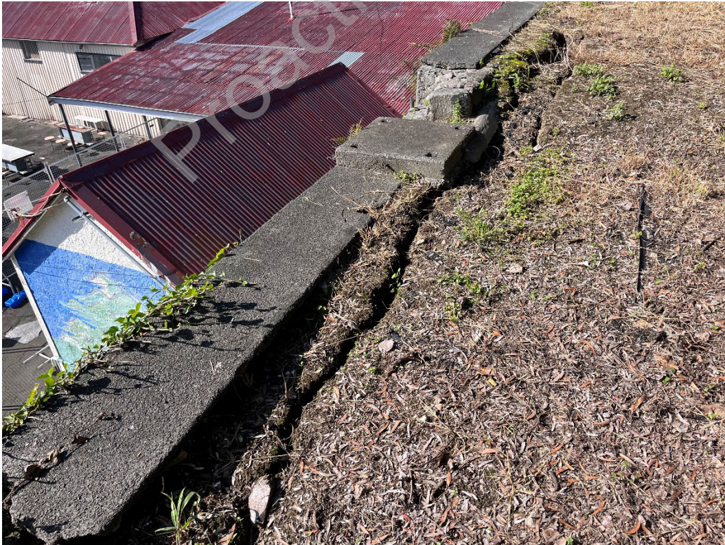
Photo 2 – Tension cracks behind RW10. Photo taken 03.03.23, looking southeast.
