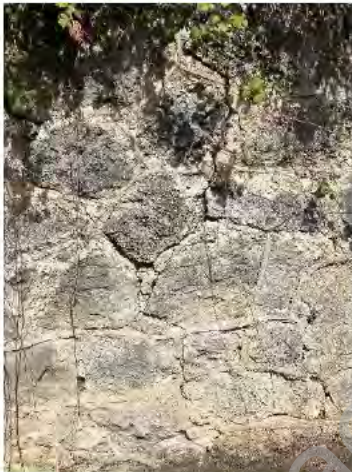
Photo 3) Cracking observed in wall face.
