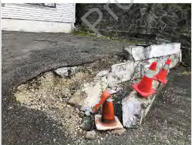
Photo 5) Erosion, wall collapse and broken top barrier.
