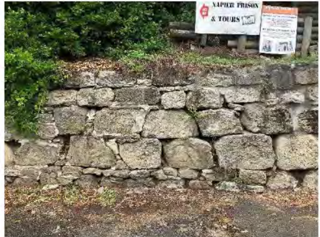
Photo 2) Loose, dislodged blocks.
