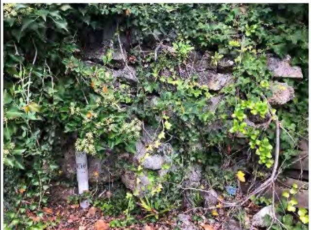
Photo 2) Heavily vegetated wall face with loosely stacked blocks.
