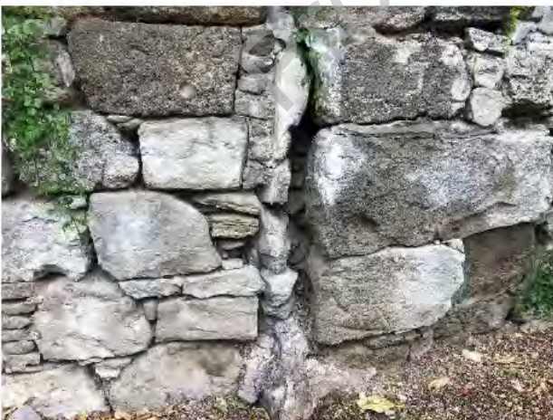
Photo 5) Large displacement/gaps observed in wall. Note old tree root at toe of wall.
