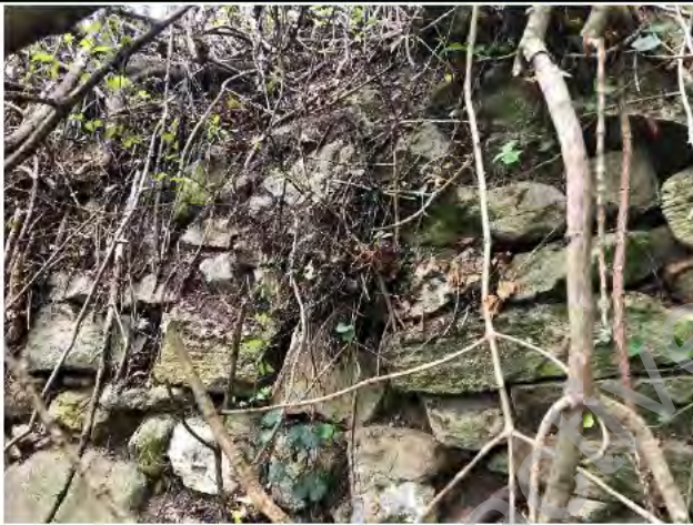
Photo 3) Loose blocks and partial wall collapse.
