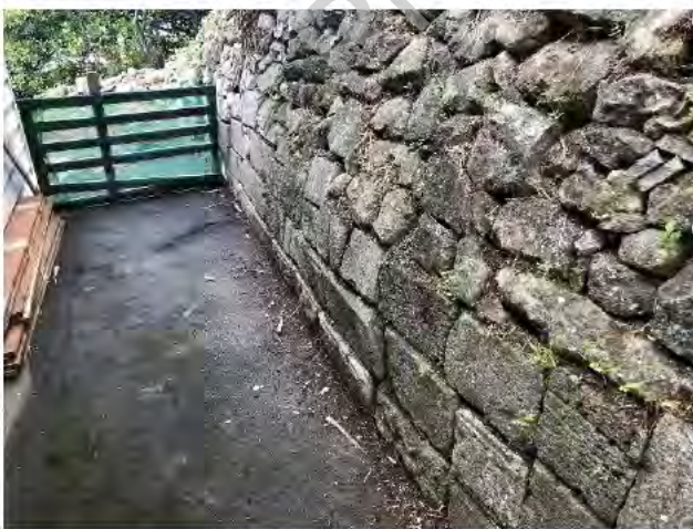
Photo 5) Bulging of wall observed.
