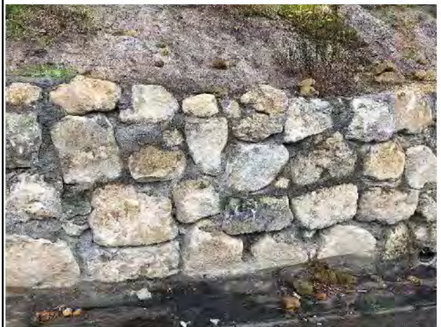
Photo 2) Cracked and missing mortar between blocks.
