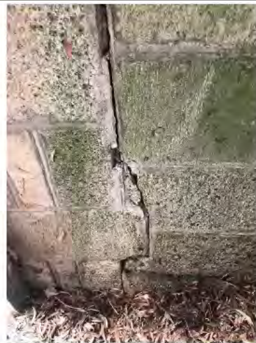
Photo 6) Cracking observed at base of wall.
