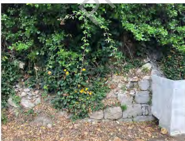
Photo 5) Evidence of old block wall, which has collapsed and eroded.
