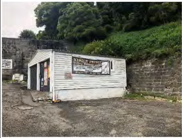
Photo 2) NAP-PRIS-08 view. Note heavy vegetation at top of wall.
