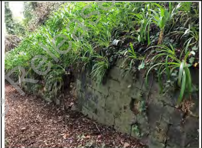
Photo 4) Cracking and partial collapse of wall observed.
