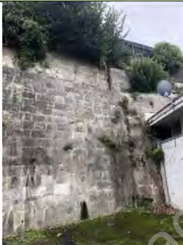
Photo 3) Vegetation and observed water seepage over wall face.
