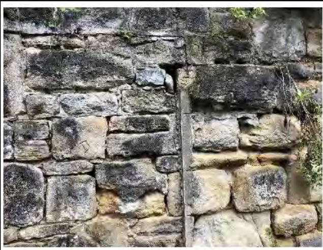
Photo 6) Erosion of stone blocks and mortar observed.
