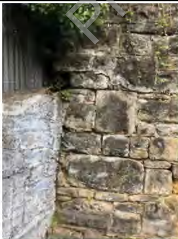
Photo 5) Erosion of stone blocks and mortar observed.
