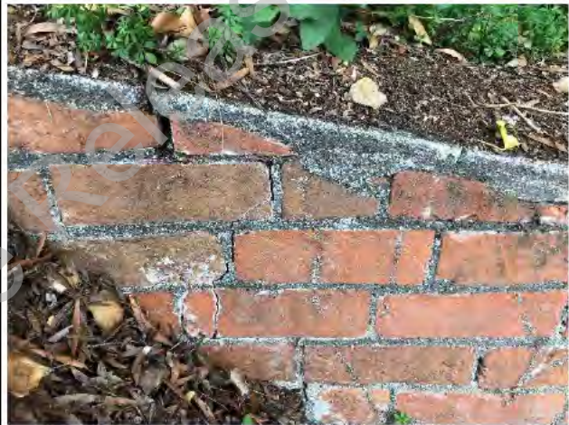
Photo 4) Cracking observed in brick masonry.
