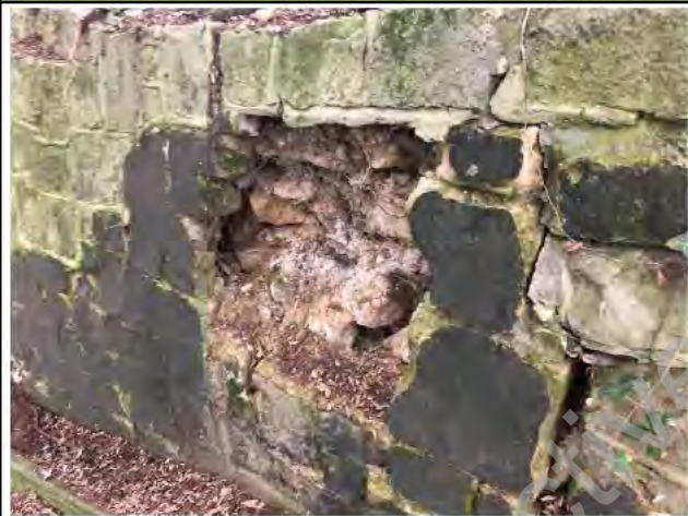
Photo 3) Cracking and partial collapse of wall observed.
