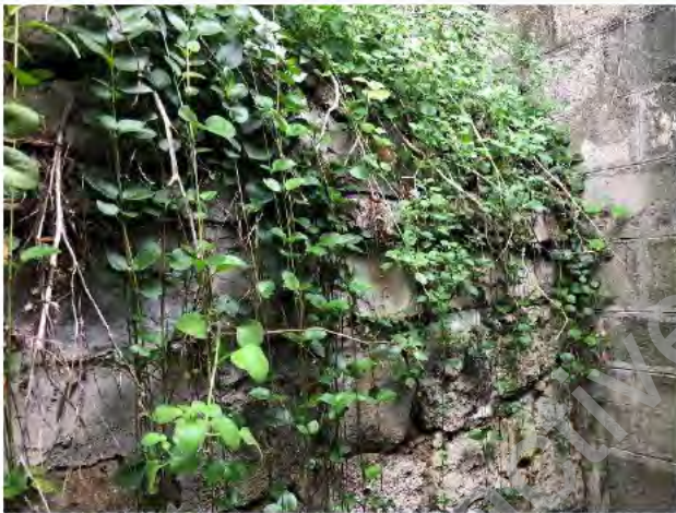
Photo 3) Vegetation observed at top of wall. Cracking and erosion of mortar and blocks.
