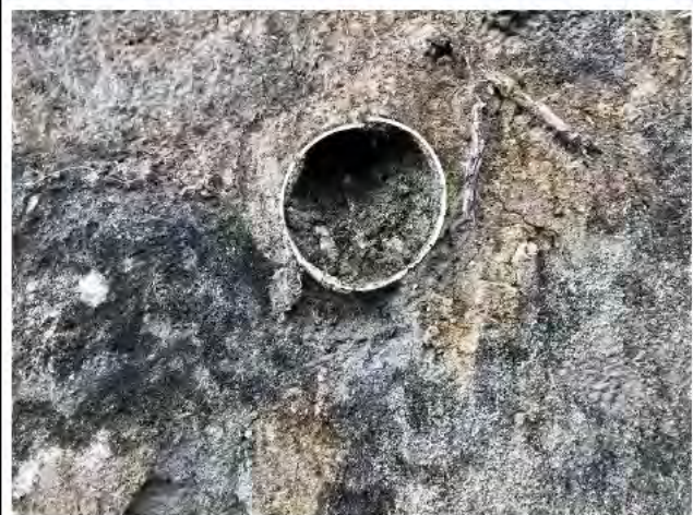
Photo 6) Weep hole, possibly recently installed, clogged with soil.
