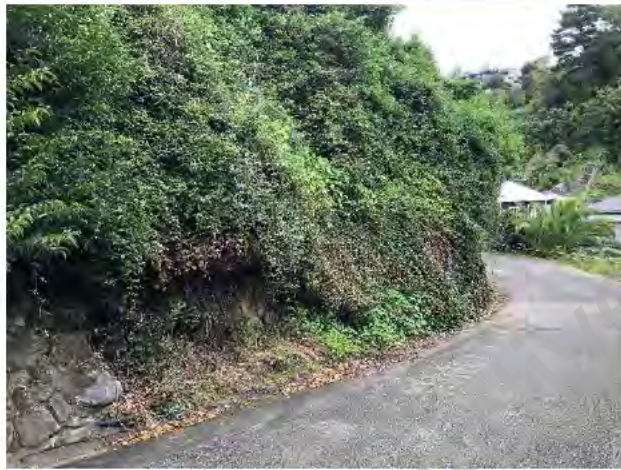
Photo 3) Significant vegetation over face of wall/exposed soils. Note steep head slope.
