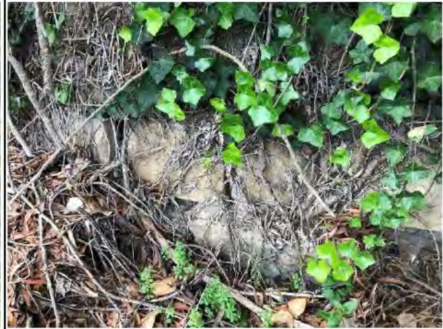
Photo 2) Loose blocks, heavy vegetation and partial collapse observed.
