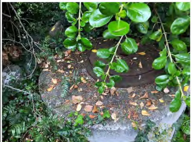
Photo 6) Manhole observed immediately behind top of wall.
