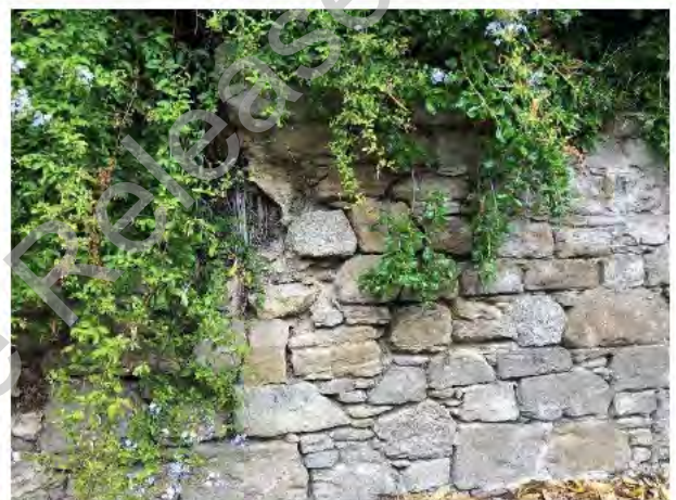
Photo 4) Collapsed section of wall with visible root growth behind wall
