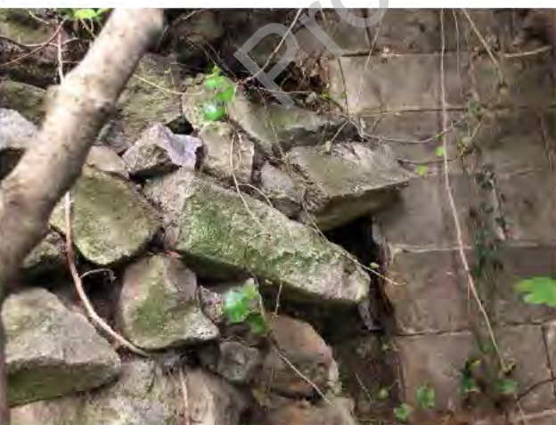
Photo 5) Interface between loose stone section and concrete block section. Note large void.
