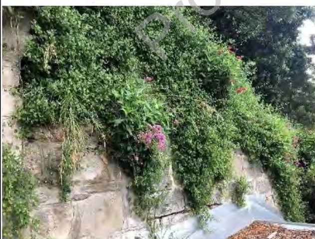
Photo 5) Cracking and vegetation growth through wall face.
