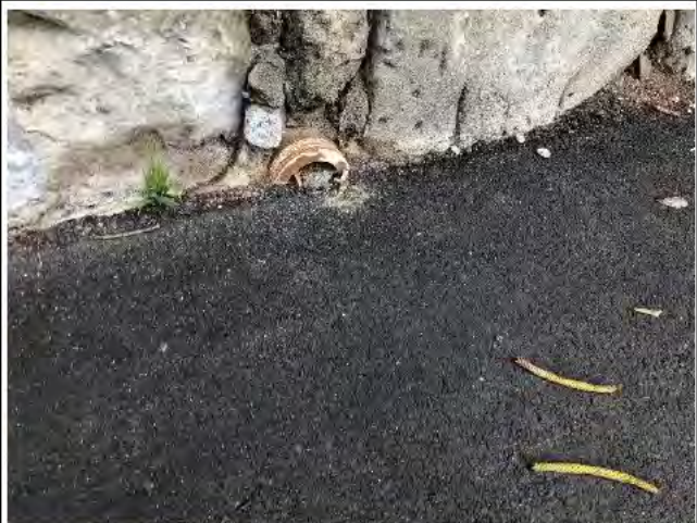
Photo 6) Old drainage pipes appear to have been recently asphalted over in places.
