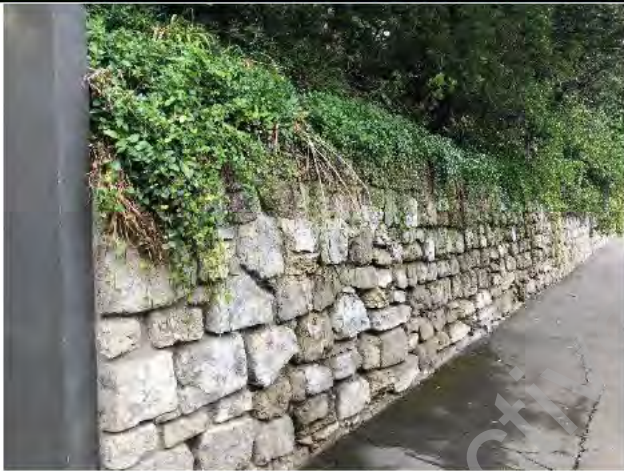
Photo 3) Loose blocks/mortar eroded between blocks.
