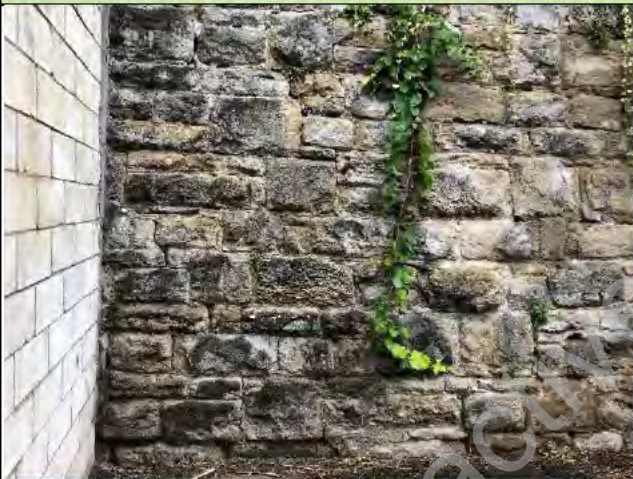
Photo 3) Cracking observed in wall face.
