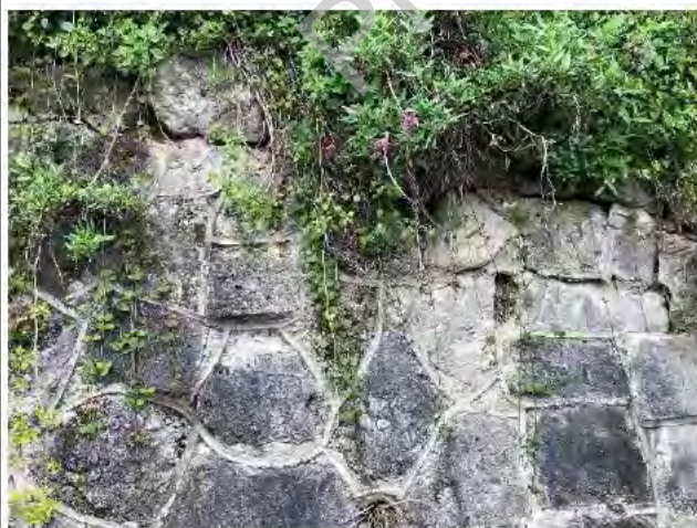
Photo 5) Cracking at top of wall where heavy vegetation present. Root growth through drains.
