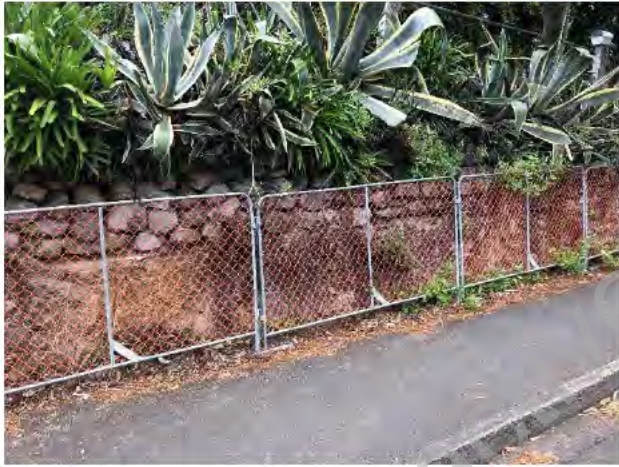
Photo 3) Loose blocks and partial collapse of wall.
