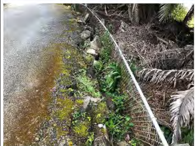
Photo 6) Vegetation and partial collapse of wall.
