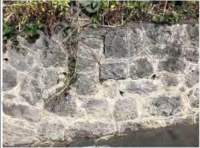
Photo 4) Cracking observed in wall face.
