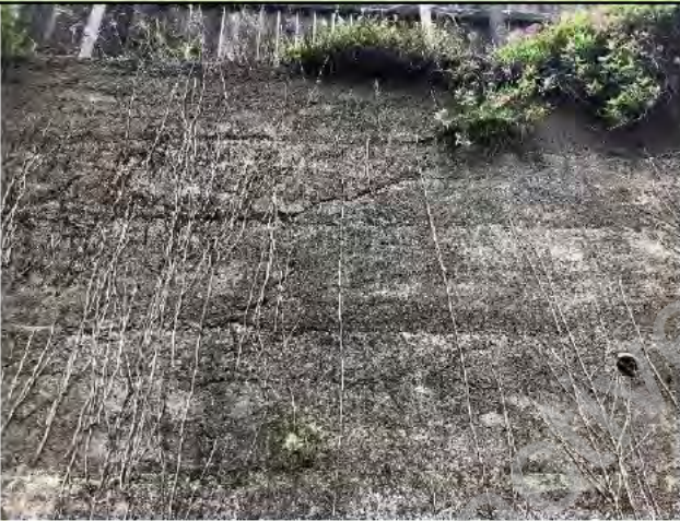
Photo 3) Some cracking observed in wall face.
