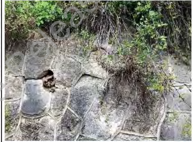
Photo 4) Cracking and broken drainage pipes observed.
