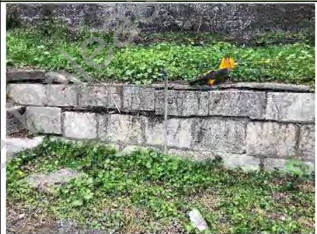
Photo 4) Loose/dislodged blocks observed.
