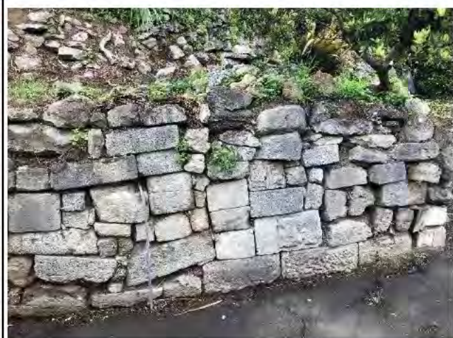
Photo 6) Loosely stacked rocks of wall face.
