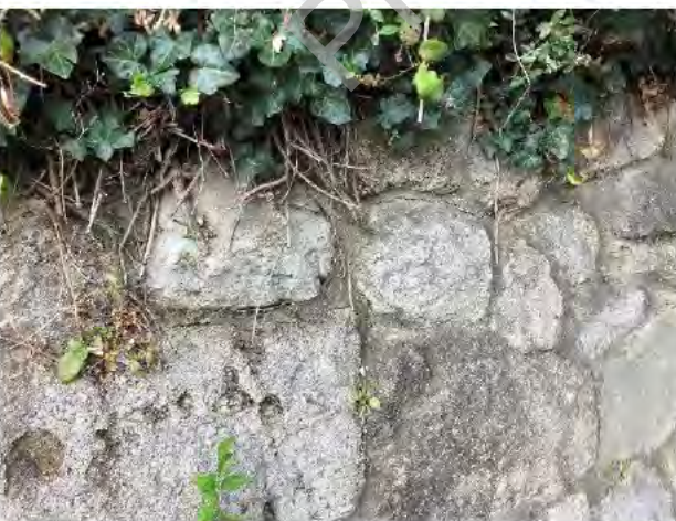
Photo 5) Cracking observed in mortar between blocks.
