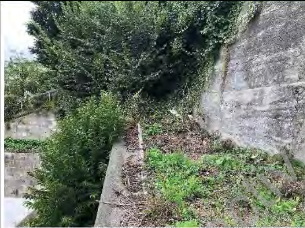
Photo 3) Heavy vegetation above top of wall.
