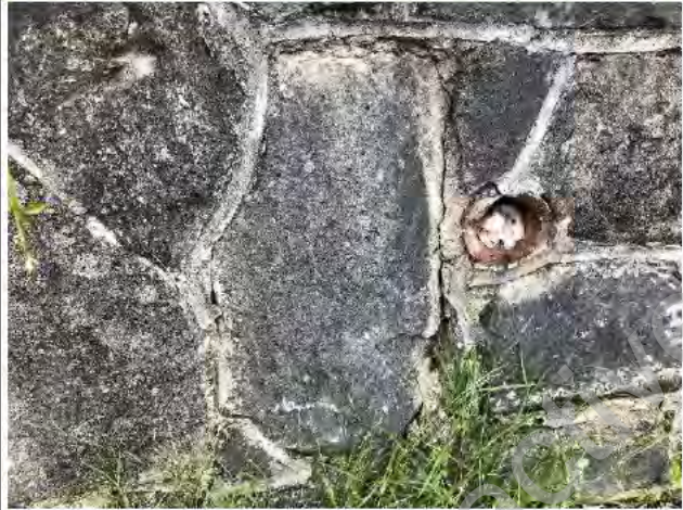
Photo 3) Cracking observed around blocks.
