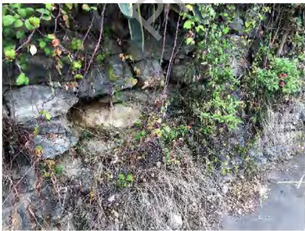
Photo 5) Loose blocks, erosion and vegetation observed in wall face.
