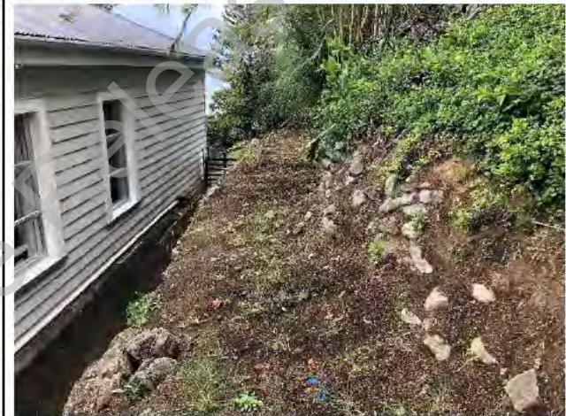
Photo 4) Top tier of wall almost completely collapsed.
