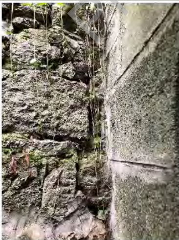
Photo 5) Cracking observed at end of wall.
