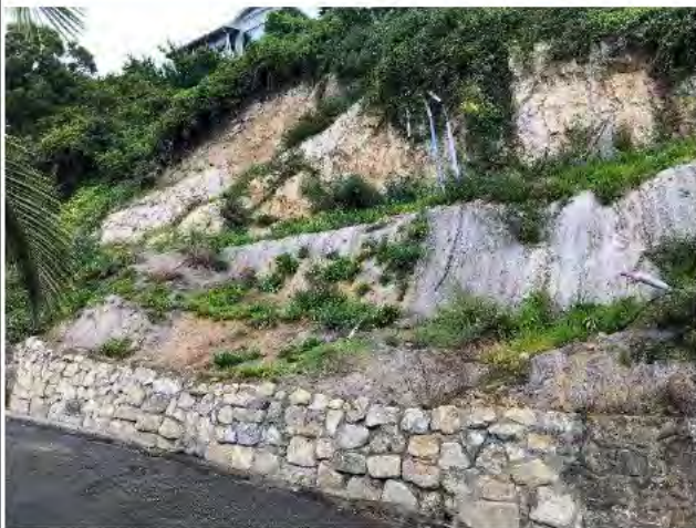
Photo 1) NAP-PRIS-06 view. Note recent slope failure and “new” construction of wall, also upslope residential property.
