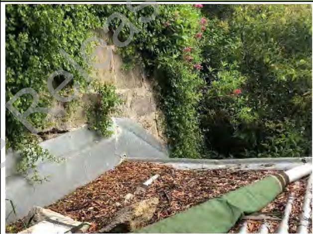
Photo 4) Cracking and observed in wall face.
