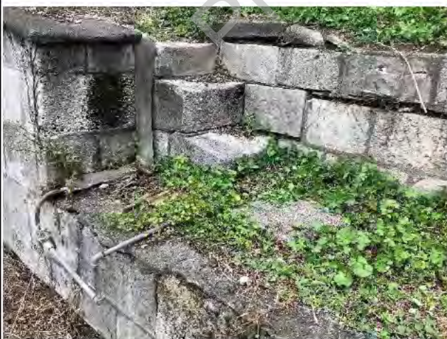
Photo 5) Loose/dislodged blocks observed. Possible wall settlement resulting in "gap".
