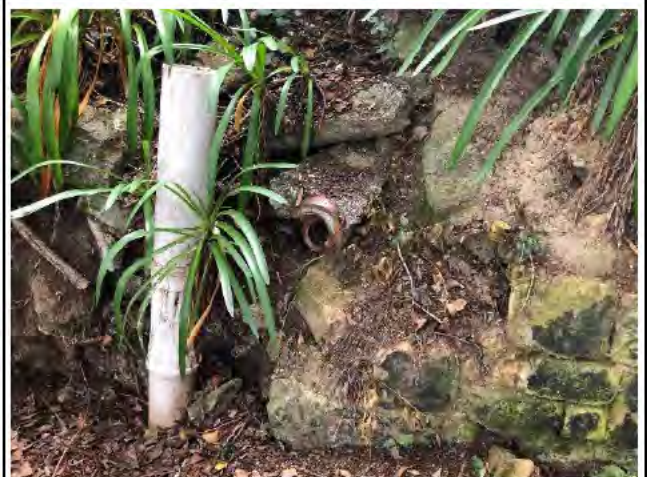
Photo 6) Collapsed section of wall immediately upslope of sewage leak.
