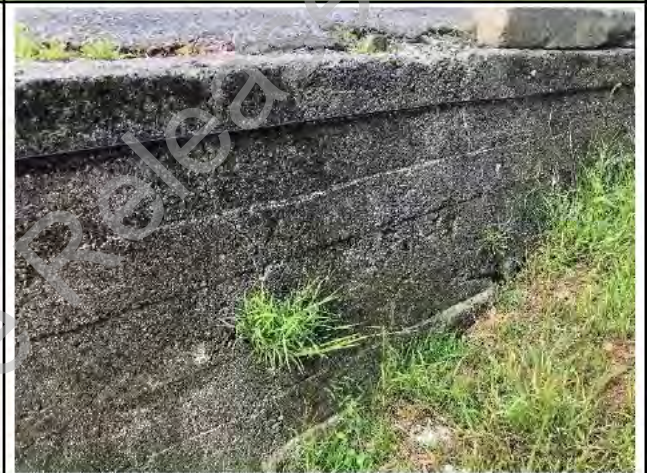
Photo 4) Cracking observed in wall face.
