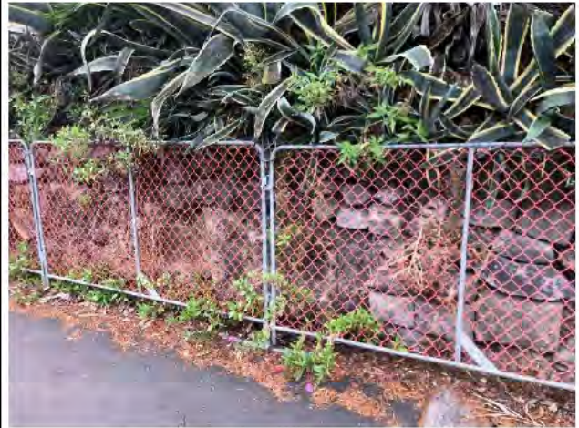
Photo 2) Loose, dislodged blocks and partial collapse.
