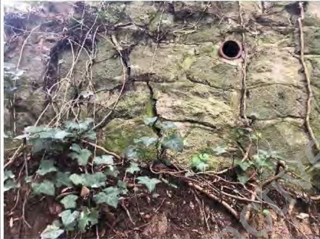
Photo 3) Cracking observed in wall face.
