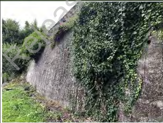
Photo 4) Vegetation growth over face.
