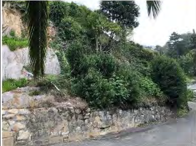
Photo 2) NAP-PRIS-05 view. Note heavy vegetation above wall.
