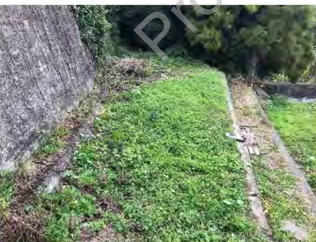
Photo 5) Toe of wall. Note exposed lip of wall toe, possibly indicating some ground settlement.
