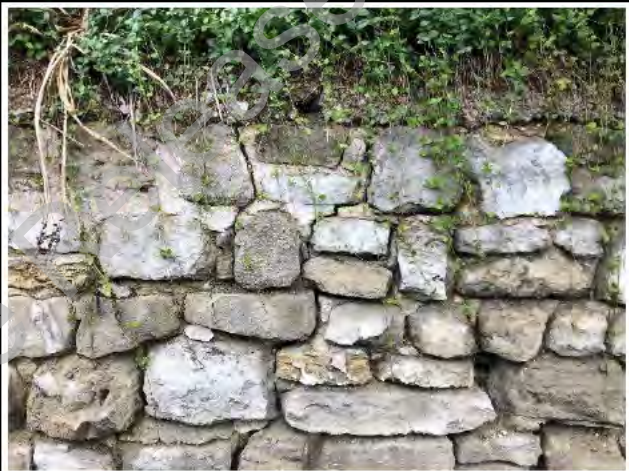
Photo 4) Cracking observed between stone blocks.
