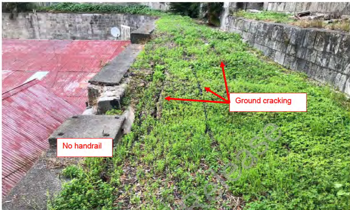
Figure 1. Ground cracking observed behind NAP-PRIS-RW10
