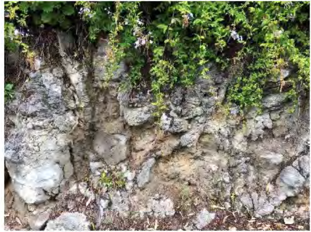
Photo 2) Exposed soil face showing evidence of erosion.
