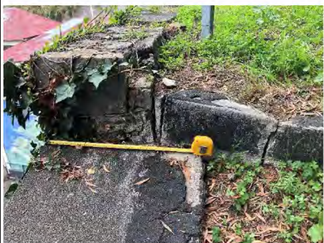
Photo 6) Cracking and possible rotation observed at top of wall.
