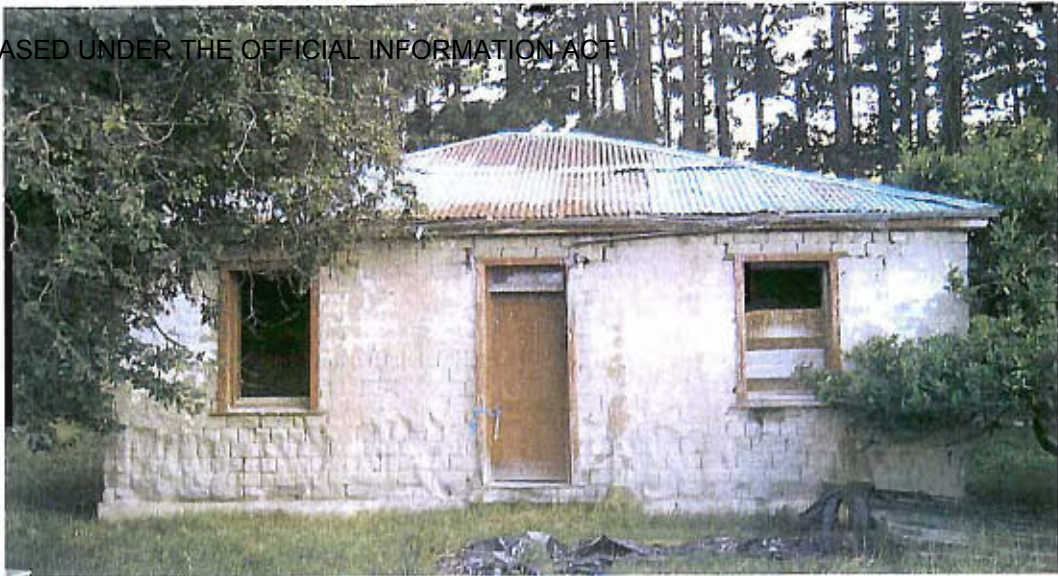
Photo 16: This mud-brick house (site 8) can be considered uncommon in Otago due to its unusually good preservation and that it is an excellent example of an early pastoral farming structure in region.
