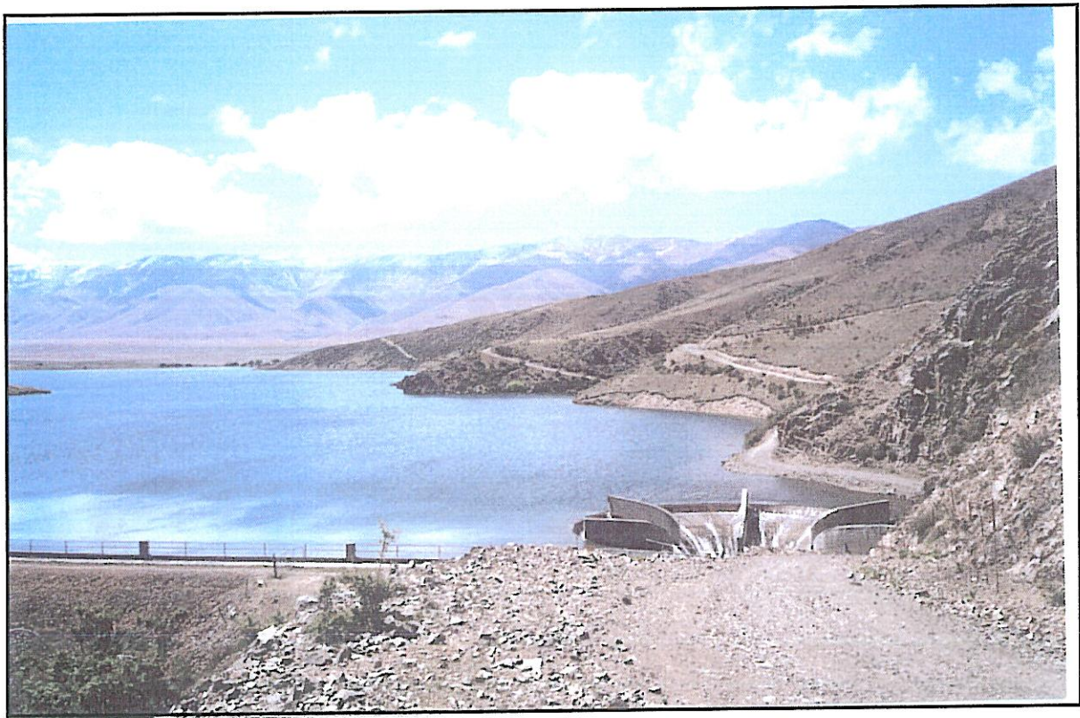
Falls Falls Dam showing part of dam wall & glory hole. Home hills on right
