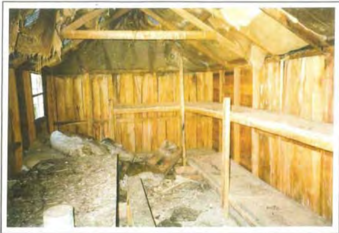
Fig. 17 The interior of this hut is currently in a semi-derelict state, but the structure appears sound and the shelter would be welcome in adverse weather conditions. It would not be difficult to restore the hut to a habitable condition and it could become a significant recreational asset.
