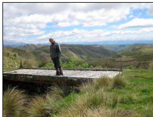
Plate 20. Old wooden bridge at GPS 006 leading to Mitchell's Hut. View north (John Barkla in photo).
