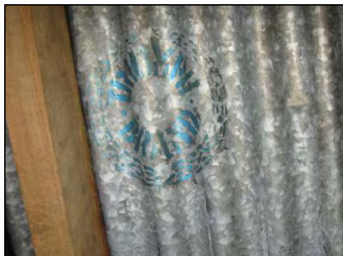
Plate 2. Triumph maker's mark on underside of corrugated iron roofing (Mitchell's hut).
