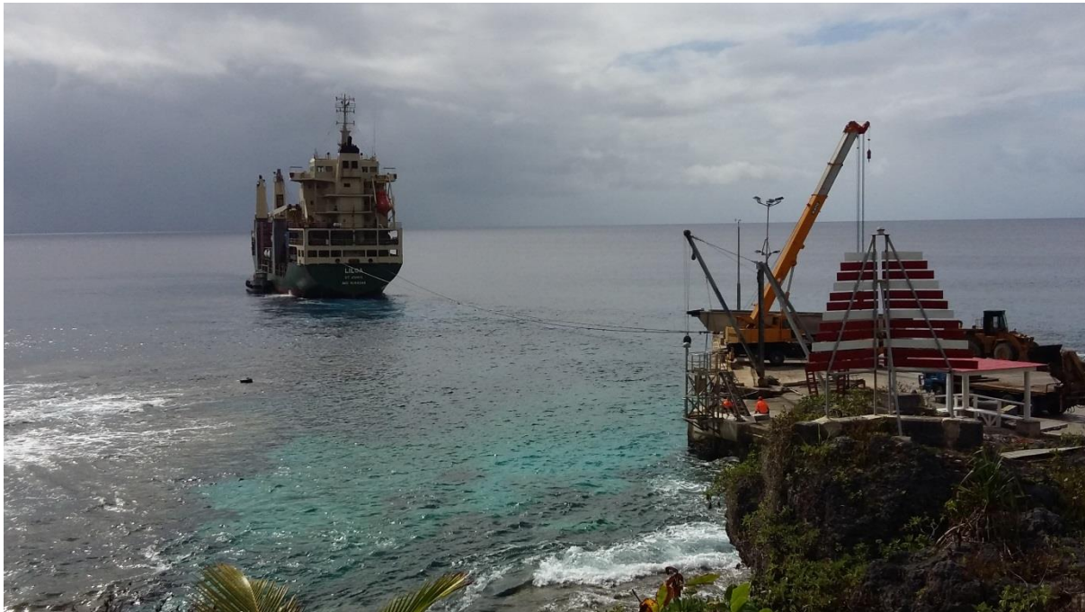
Figure 13: MV Liloa moored at Alofi, note mobile crane on wharf preparing to launch barge
