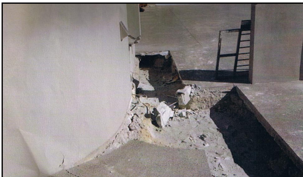
Figure 5 – Displacement due to liquefaction (Photo- Eliot Sinclair and Partners)
