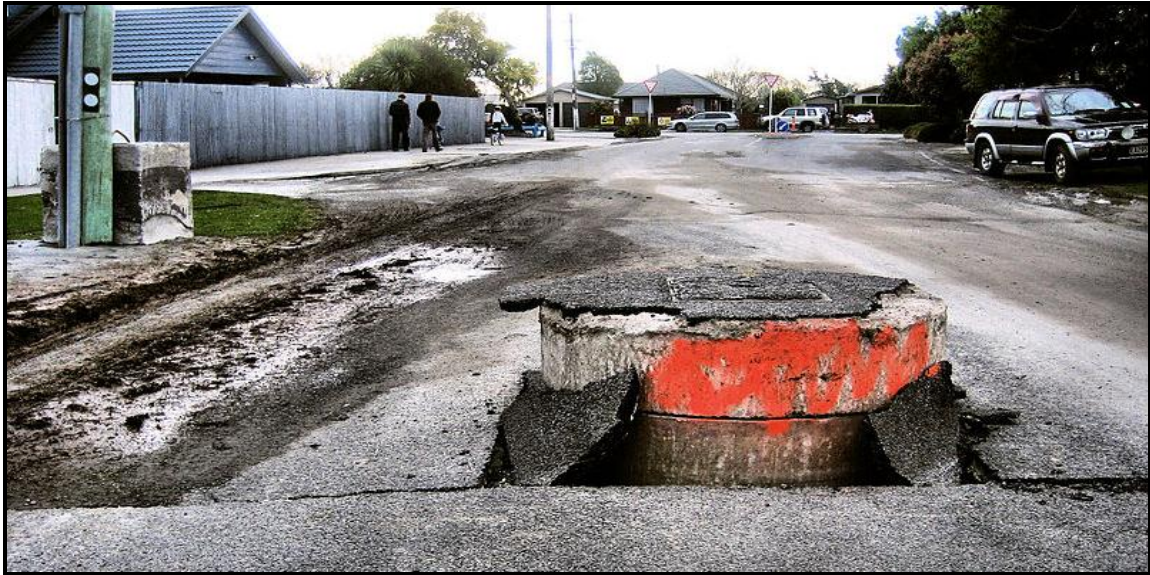
Figure 2 – A storm water manhole raised by liquefaction (Photo - Wikipedia)
