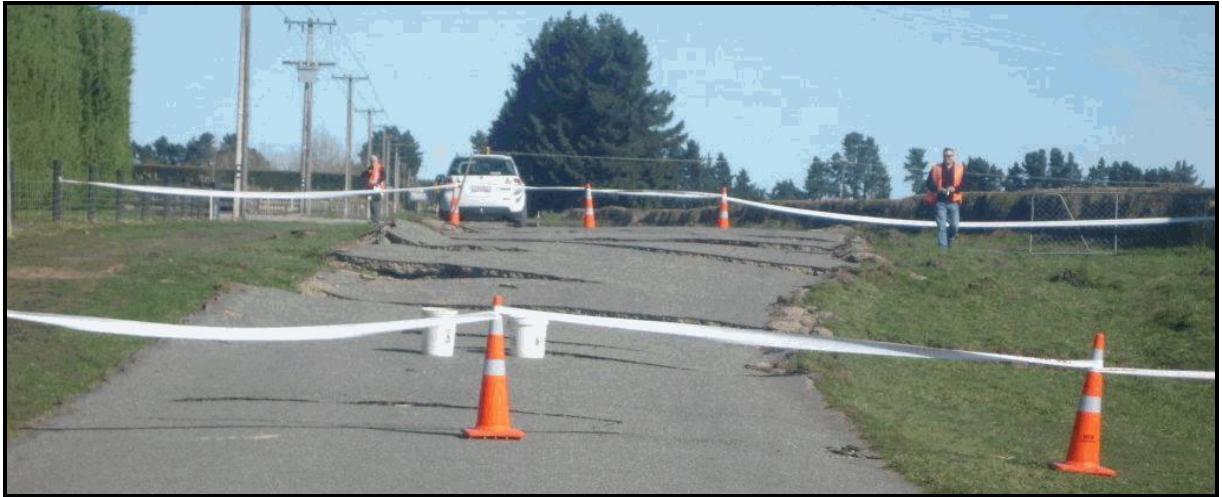
Figure 4 – Effects of fault rupture – previously straight road (Photo - Survus Consultants)
