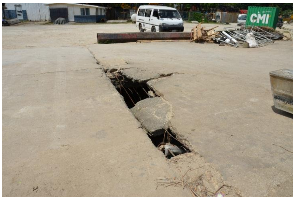
Figure 4-5 : Star Wharf is in a Deteriorated Condition
