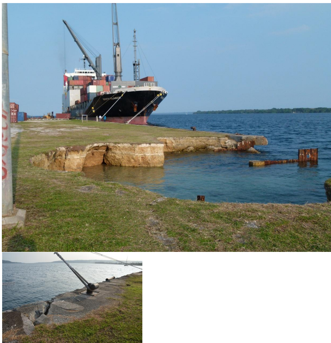
Figure 7-1 : Mooring Bollards Need Upgrading at Main Wharf, Luganville for Large Vessels The Berth has been Undermined and Washed out at its Eastern End.
