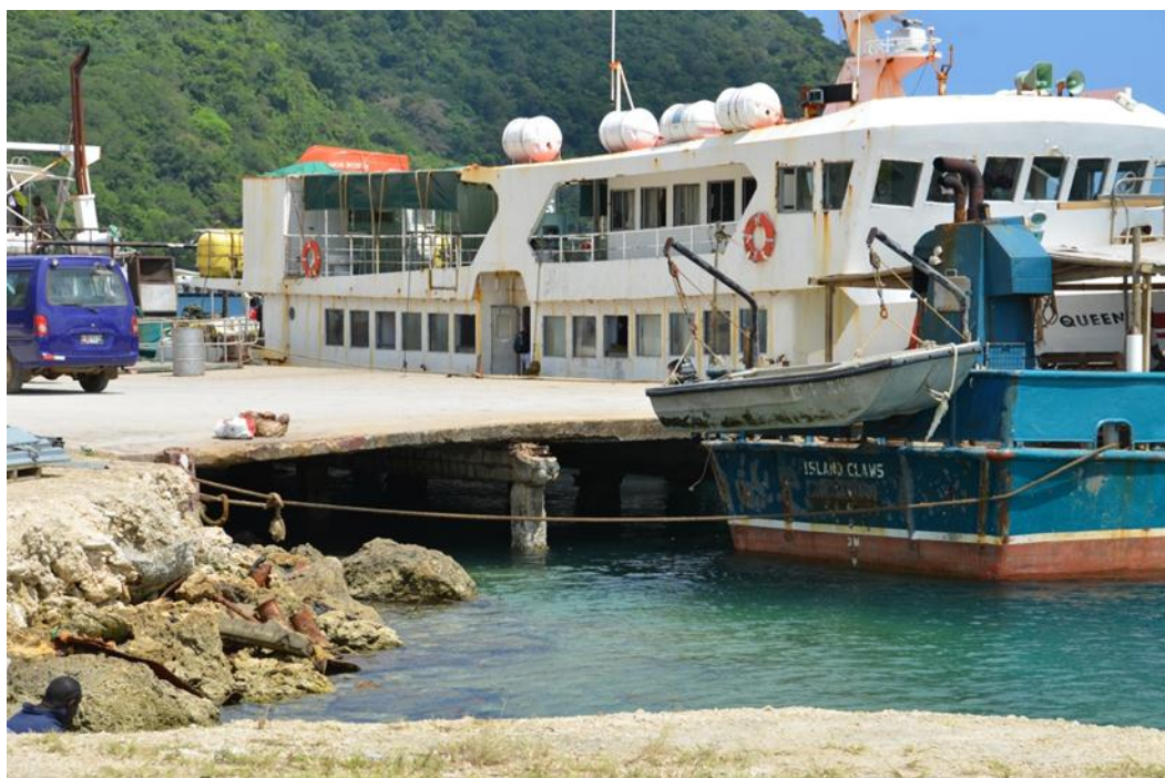
Figure 4-4 : Star Wharf is of Light Construction and in Poor Condition
