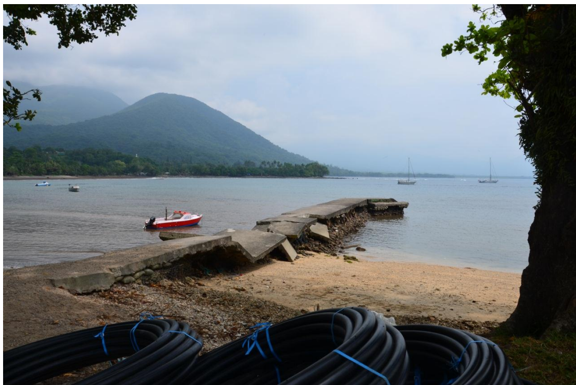
Figure 4-2 : Jetty at Sola, built in 1997. Undermined and Damaged by a Cyclone, 2011
