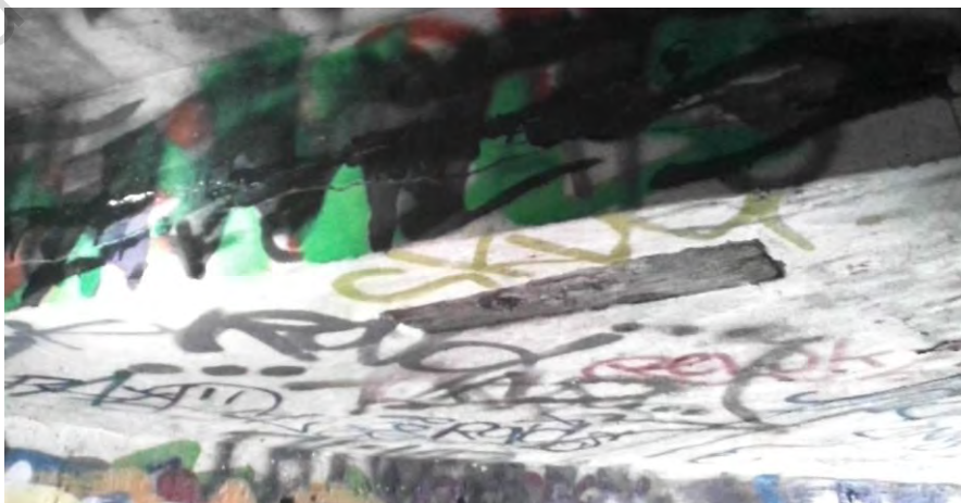
Figure 6 – Crack in 6" artillery store roof soffit
