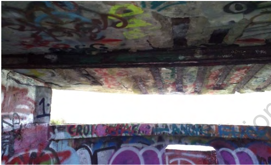
Figure 8 – OP Roof Corrosion
