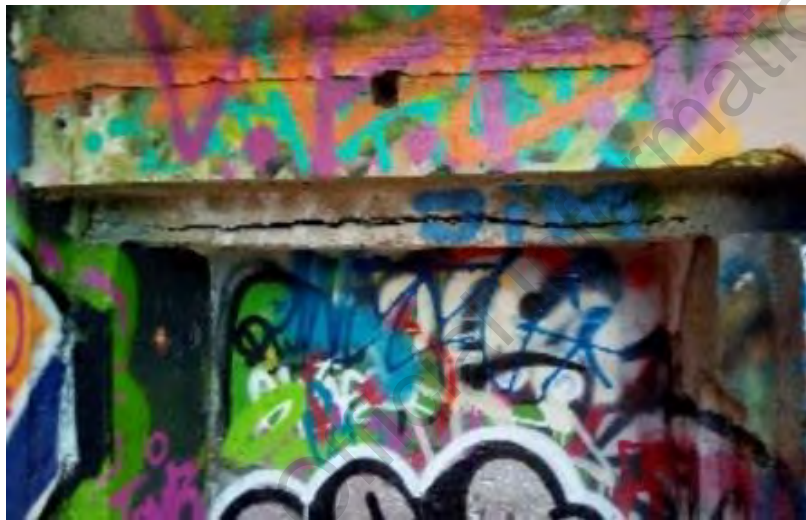
Figure 7 – Crack in 6" gun pit horizontal door crack
